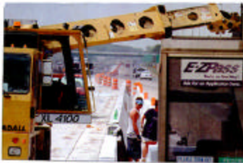
Workers install a high-speed E-ZPass lane at the Dover toll plaza. The project will include a new toll plaza, a new toll booth and a new toll plaza. The project will include a new toll plaza, a new toll booth and a new toll plaza.
